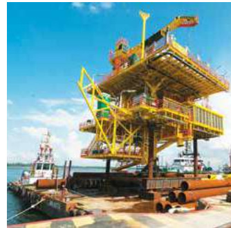
→ Offshore Wellhead Facilities (OWF) Tembikai Non-Associated Gas (TNAG)
